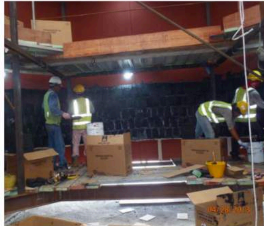
Picture 3: Pennguard application from a scaffold on ground level in the erected flue
